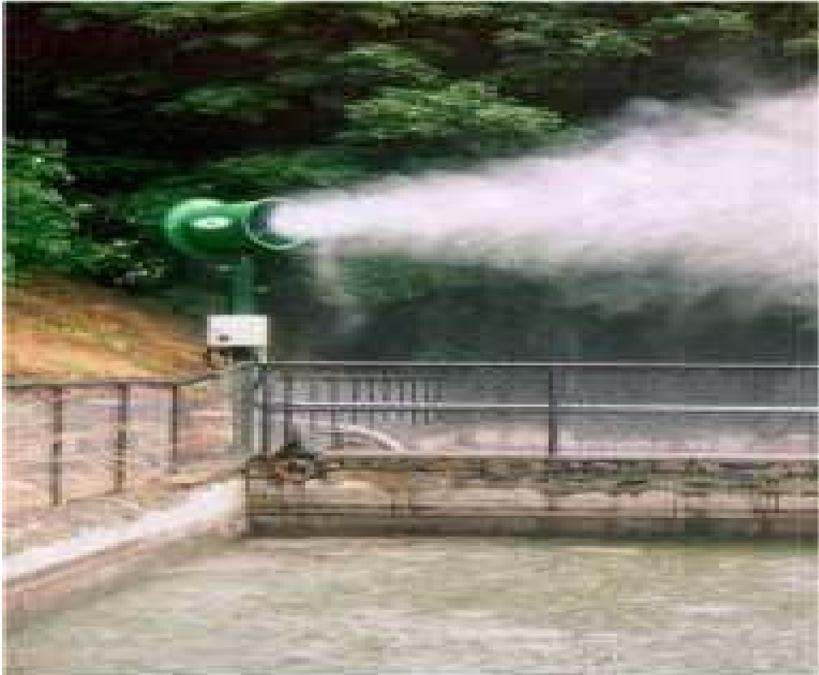
Figure 3. A typical atomizer installation for odour control
