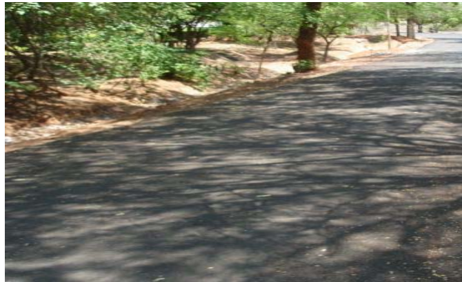
Photo : Canteen road No Pot hole
