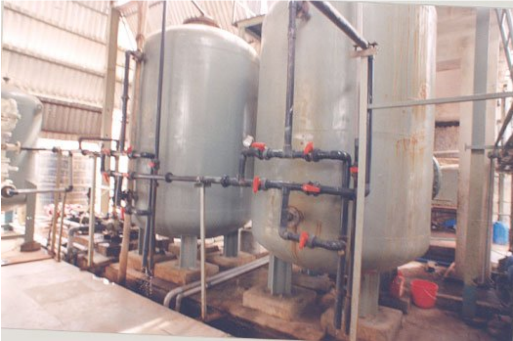
Activated Carbon Adsorption Plant
